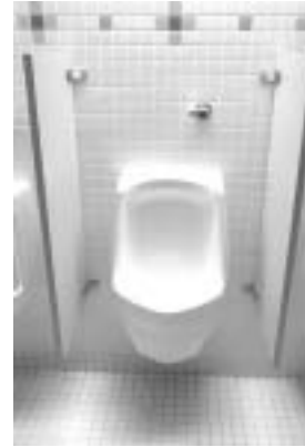
Waterless urinal installed at Seattle University
